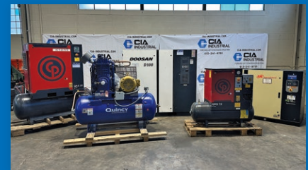
(9) Air Compressors from 100 HP to 7.5 HP
