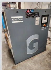
40 HP Atlas Copco GA30FF Air Compressor (2014)
