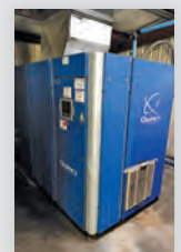
Air Compressor Systems
